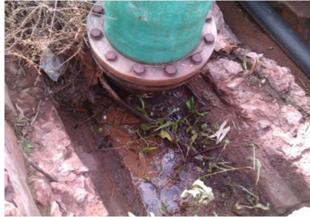
Ongoing water leak requiring action
