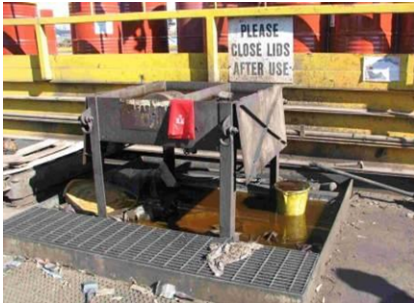
Bund requires emptying. Reduced capacity Rubbish in the bund
